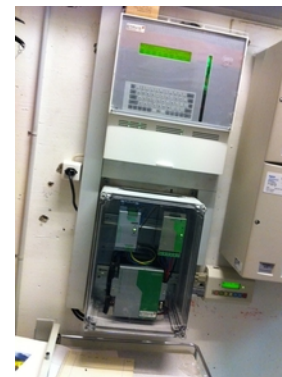
Residence St. Martin - Zentrale APS Gets
