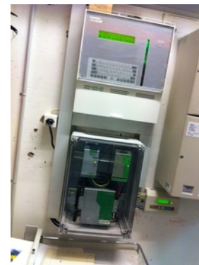
Residence St. Martin - Zentrale APS Gets
